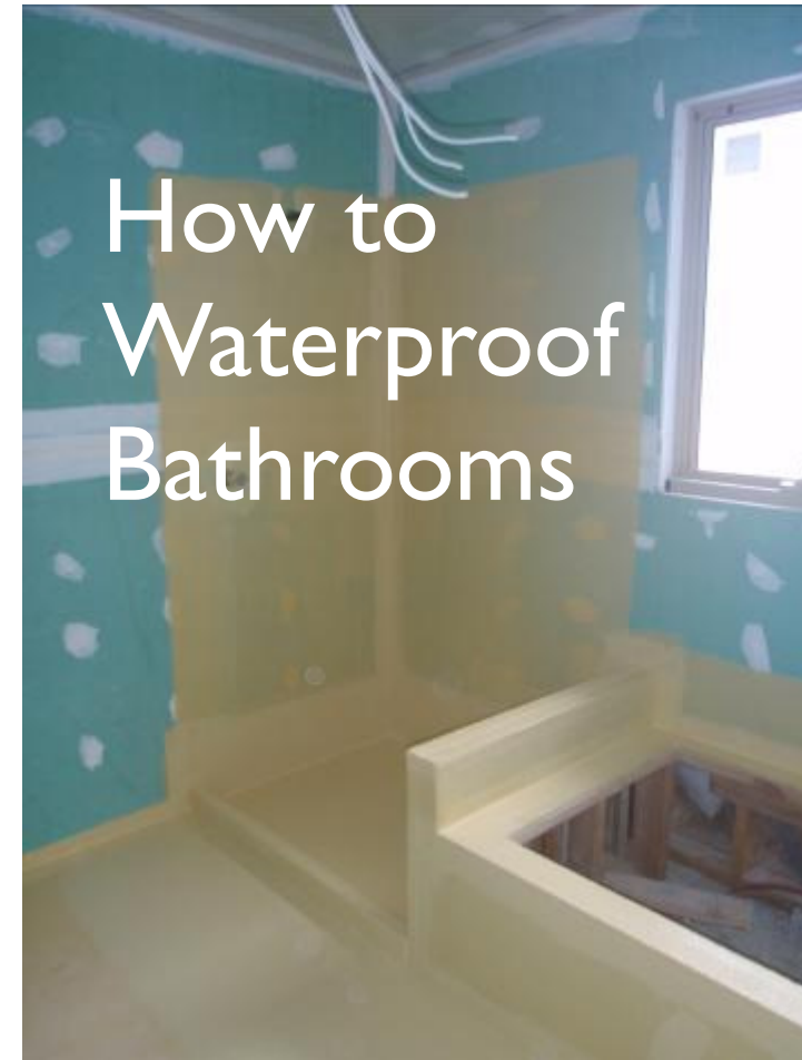
Shower zone in photo shows only one coat of membrane
