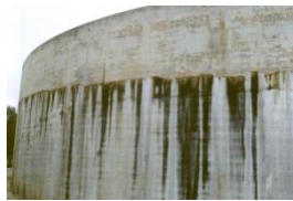
Typical construction joint problem
