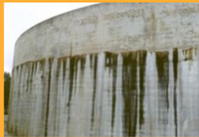
Typical construction joint problem
