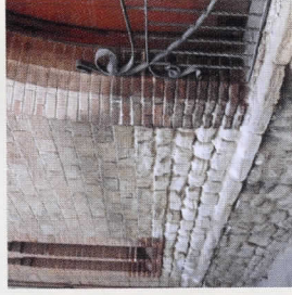
Rising damp in stone wall
