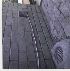
Rising damp in brick veneer wall below damp course
