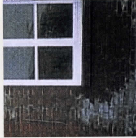
Rising damp in brick wall
